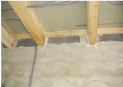
Example of a parge coat applied with scratch finish to a block wall up to internal joist level
