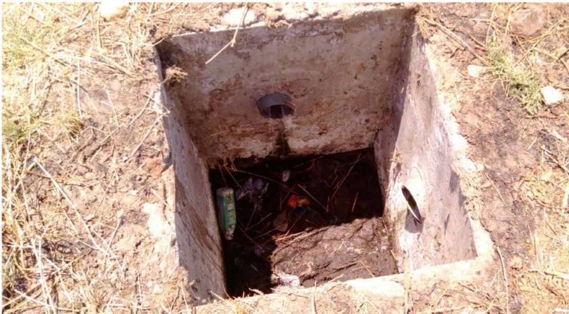
Figure 4-4: Dry non-sewer receiving manhole with solid waste
