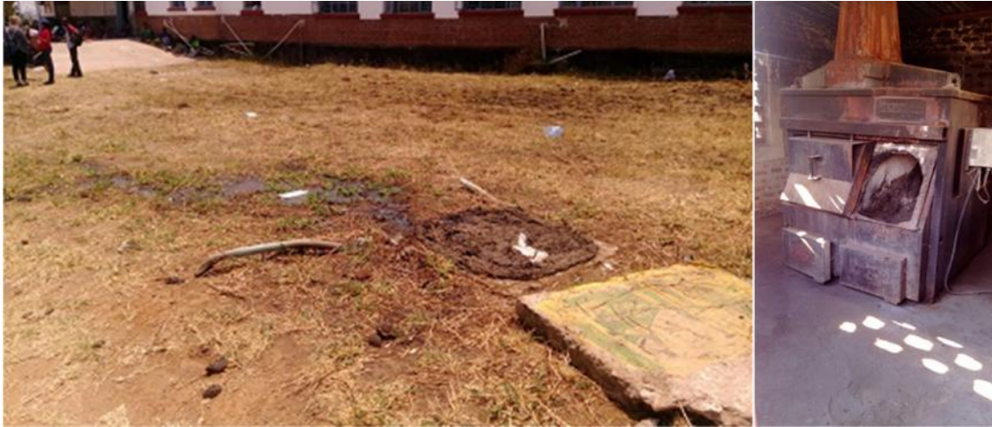
Figure 4-3: Picture site 2-blocked overflowing sewer manhole; incinerator
