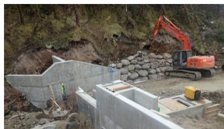
Donich Water Hydro project
