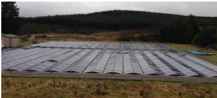
Photograph: Scottish Water's new PV scheme at Black Esk facilities.
