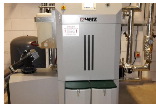
Photograph: Scottish Water's biomass boiler at Penwhirn facilities.
