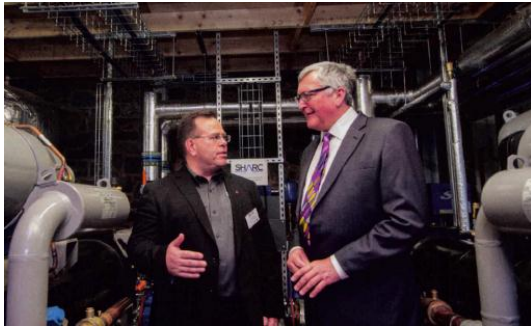
Photograph: Ross Burton – SHARC Energy (left), & Fergus Ewing MSP (right) at Galashiels facilities.
