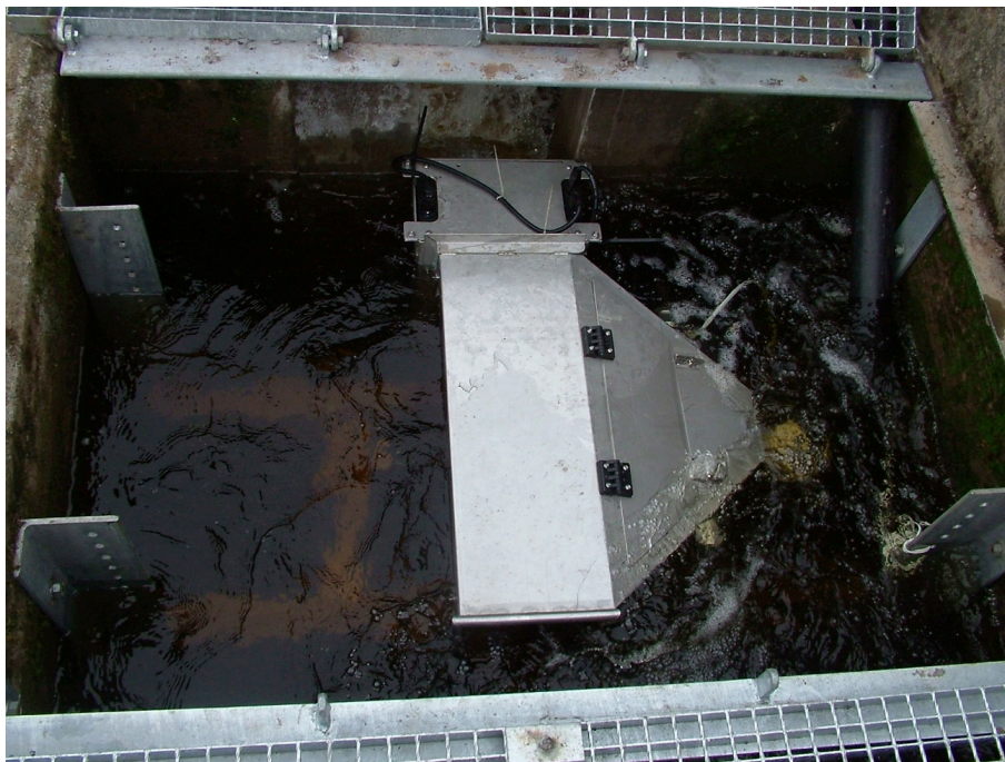
Figure 3.26. Photo of the Vaki counter and colour video camera installation at the Skinworks Cauld fish pass. Fish enter the counter at the top of the photo and exit at the bottom. The triangular section of the counter box on the right side of the photo is the colour camera and viewing window. Photo courtesy of James Hunt.
