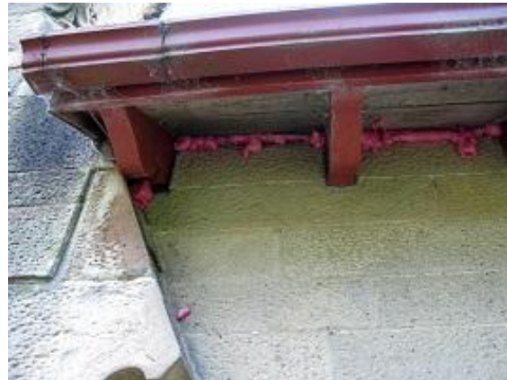
Damaged bat roost © John Haddow
