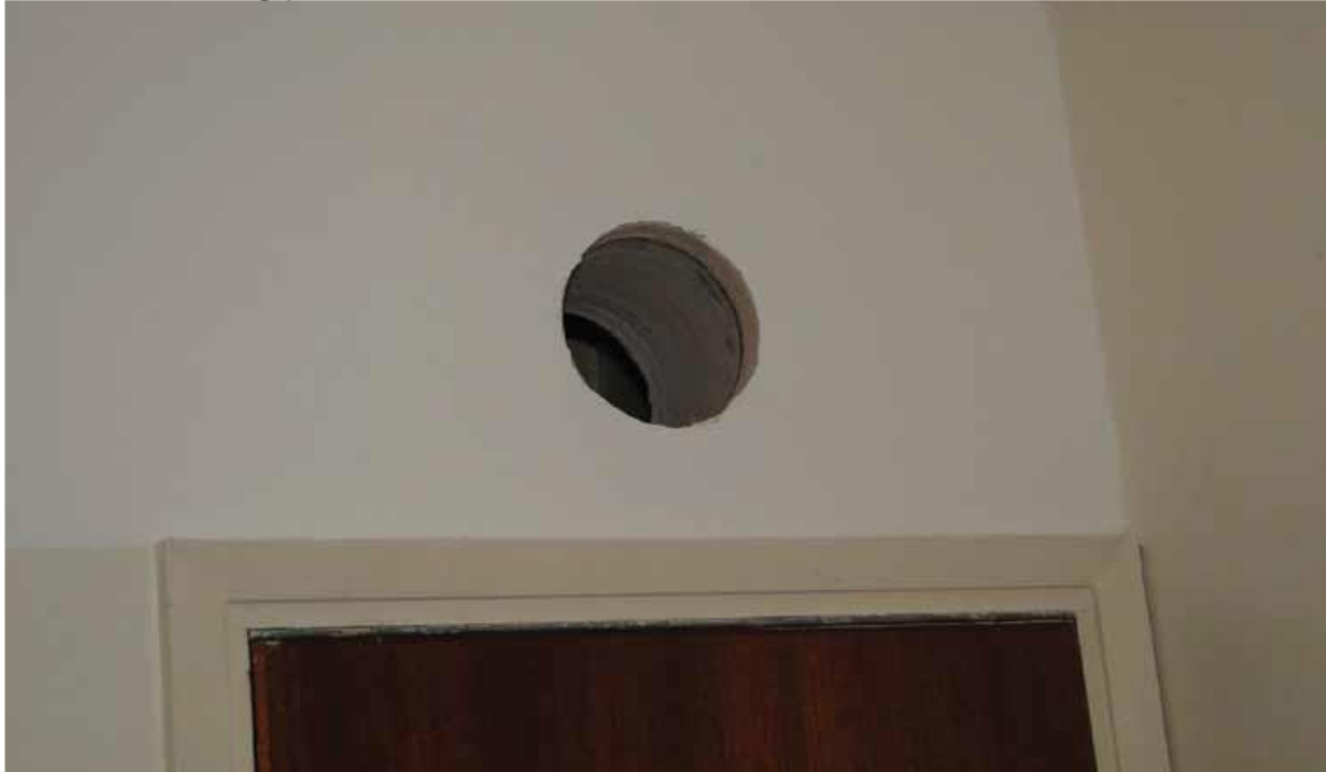
Figure 10 breach of fire-resisting enclosure
