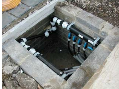
Figure 10: A typical manifold pit for horizontal loops, slinkies or bore hole systems
