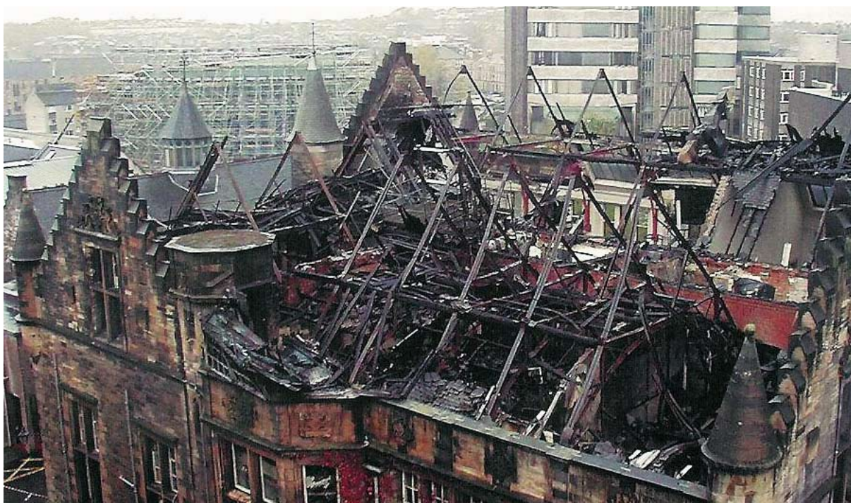
Illus 2.4.1 The presence of large, unpartitioned roof voids has resulted in severe fire damage to the roof and interior of this Category A listed university building. (Picture by Leigh Johnston, Historic Scotland and reproduced here from TAN 28).
