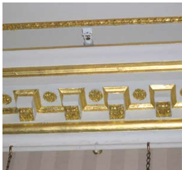
Figure 2.15.2 Sidewall sprinkler head above a cornice in Duff House. (Photo: D Urquhart).
