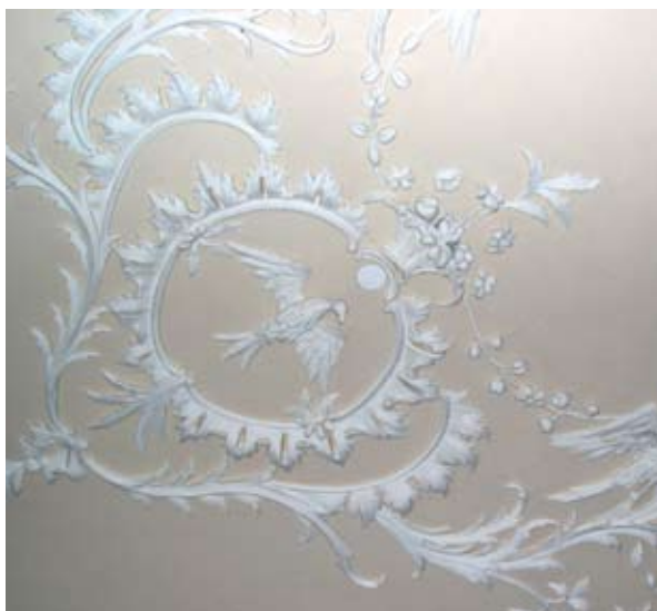
Illus 2.15.1 Discreet sprinkler head located behind a colour-matched circular cover in ornate ceilings at Duff House (Photo: D Urquhart).
