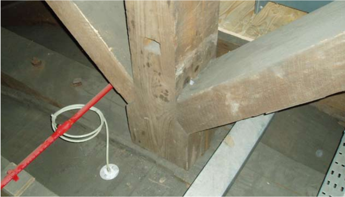
Illus 2.11.1 Installation of an aspirating smoke detector system in a ceiling void. Shown is the main plastic air pipe with an 8mm diameter tube from it to go through an 8mm hole in the roof boarding (Photo: S Brown).
