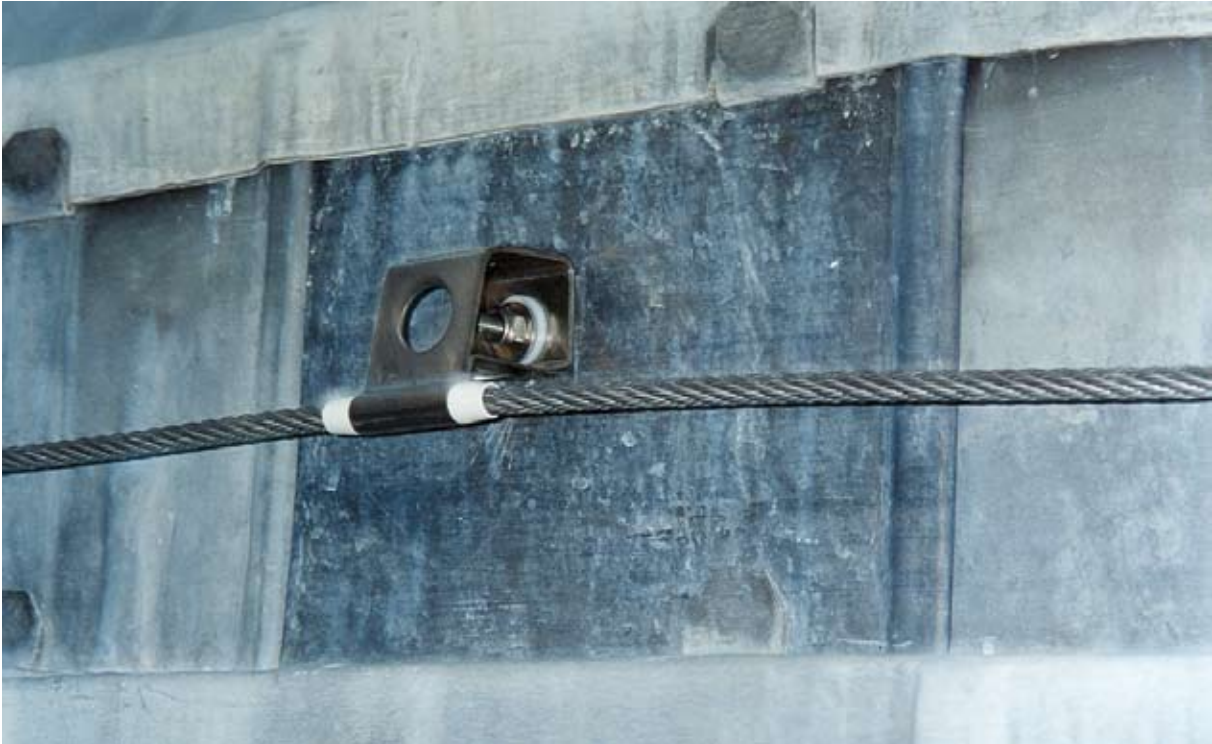
Illus 4.8.1 Continuous horizontal lifeline fixed to lead-work at General Register House, Edinburgh (Photo: J Cunliffe).
