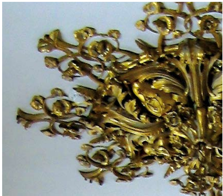
Illus 2.11.2 Very discreet smoke detector set into historic ceiling. The detector head is located to the left of the ceiling rose (Photo: I Gough).
