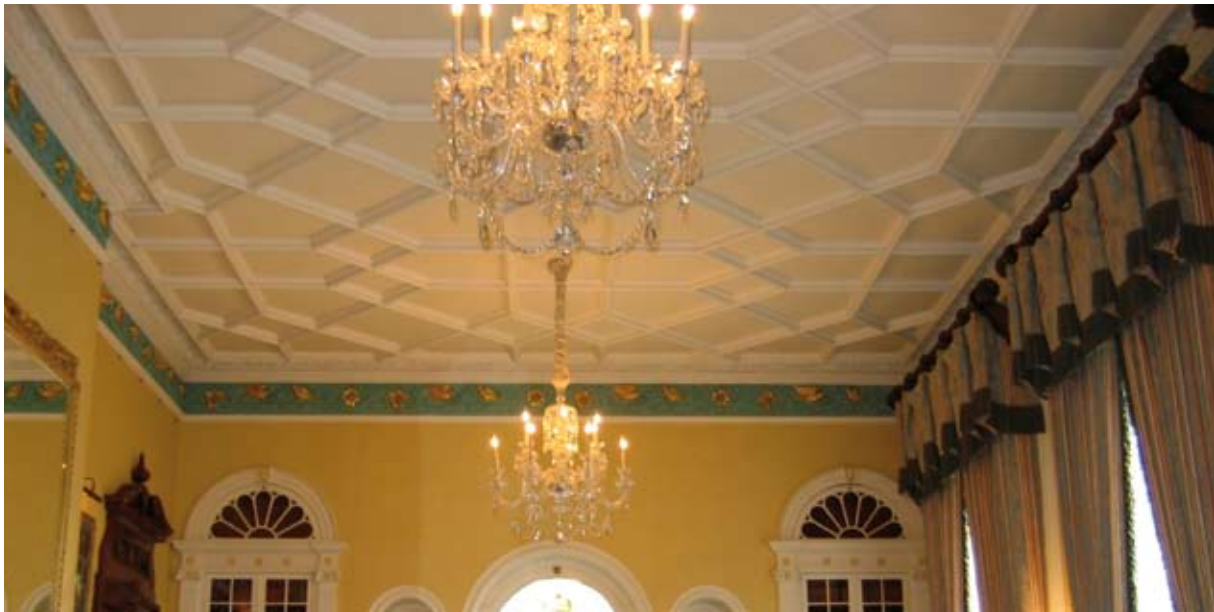
Illus 2.2.2 Historic ceiling to separating floor in a country house hotel – the ceiling has had fire resistance duration improved by the addition of intumescent paper (Photo: Ian Gough).
