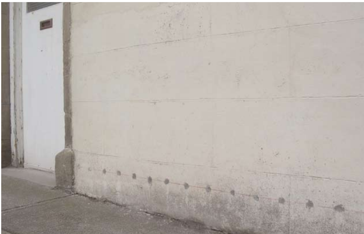
Illus 3.4.2 Damproofing inserted into a historic wall, circa mid-C19 (listed Category C(S)) (Photo: D Urquhart).
