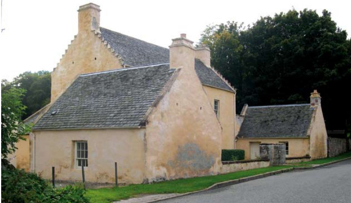
Illus 3.4.1 Dampness in a lime mortar rendered wall (Category B listed, mid-C19) (Photo: D Urquhart).
