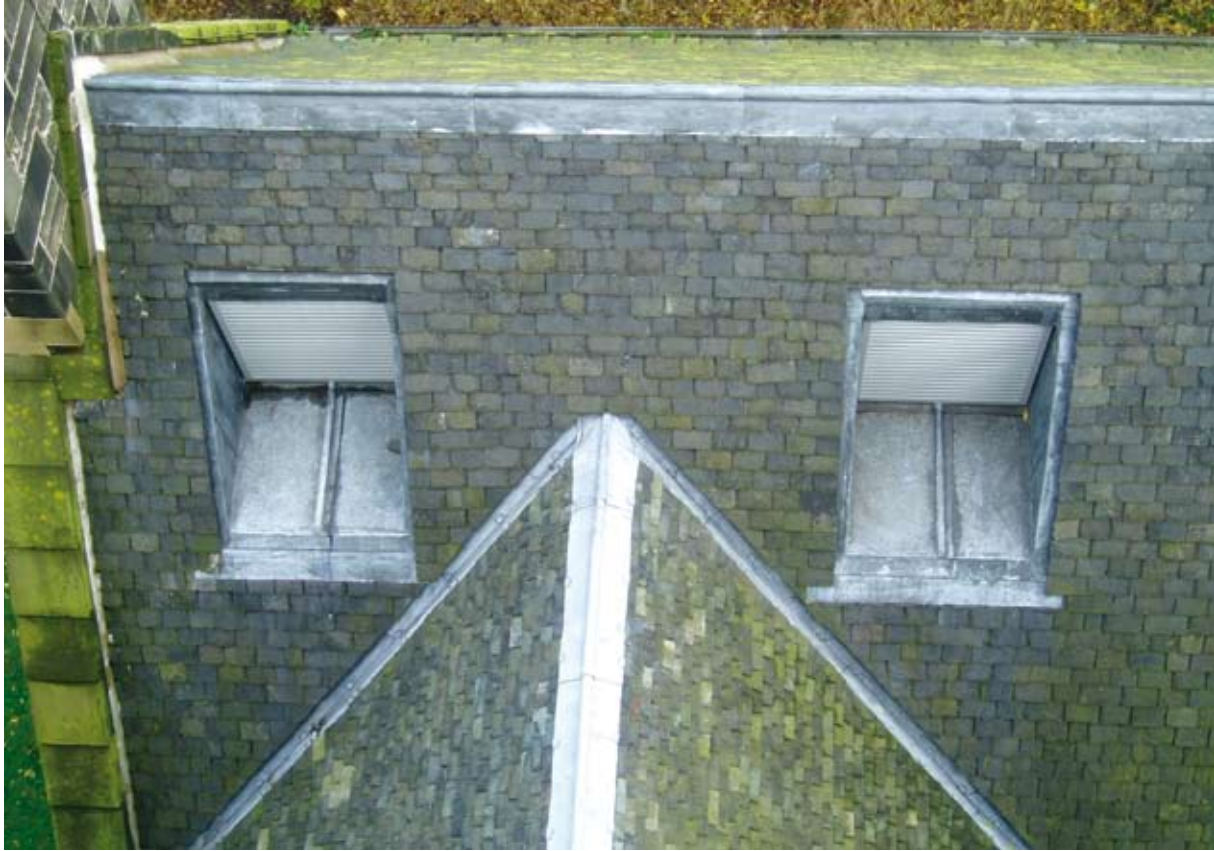
Illus 3.14.5 Inset dormer vents on a traditional pitched slated roof. Inset dormer vents eliminate the need for large, intrusive ventilation grills.
