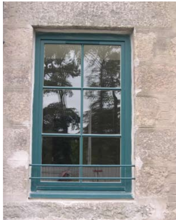
Illus 3.16.1 New window frame fixed into resized opening in this former mill converted to apartments. Note the rather poorly executed mortar pointing around the repositioned stone sill.
