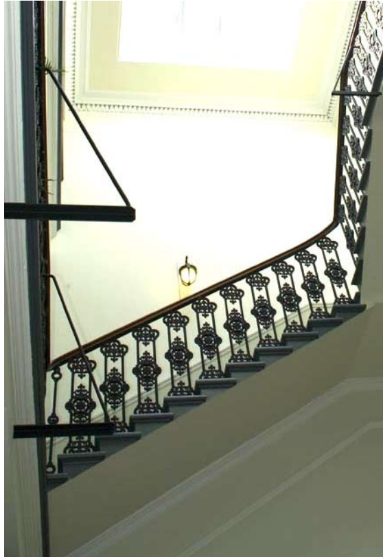
Illus 1.1.11 Fine example of cantilevered stone staircase in this former hospital converted to offices. Note the slenderness of the self-supporting stone steps and the original iron balustrade. (Photo: Historic Scotland).
