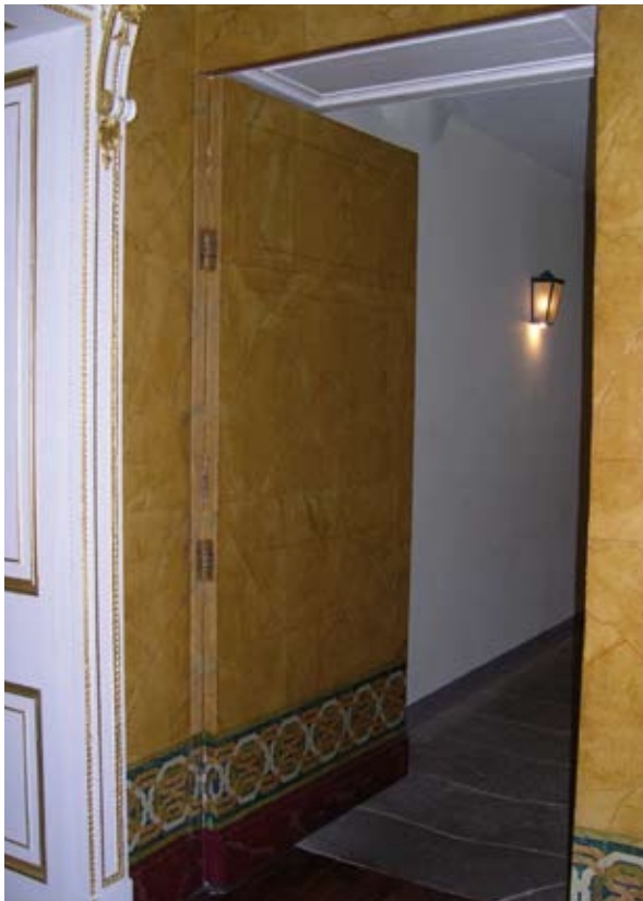
Illus 6.2 Historic (secret) door with upgraded fire resistance, in listed Category A building.
