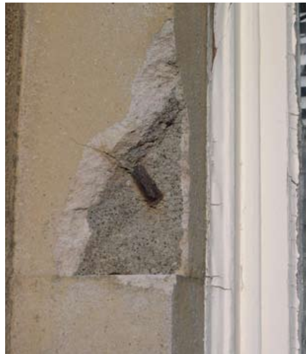
Illus 2.2 Sandstone façade repaired with precast concrete synthetic stone instead of matching stone indents. Corrosion of steel reinforcement has caused spalling of the block. (Photo: D Urquhart).
