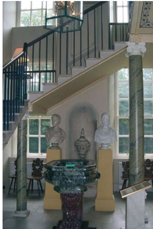
Illus 5.1 Structural support for this stair in Duff House would be difficult to determine using current design criteria (Photo: D Urquhart).
