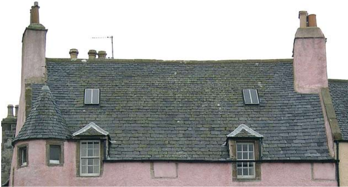
Illus 2.1 Traditional Scottish slated roof. The Scottish slates laid in diminishing courses are an important aspect of the character of the roof (Photo: D Urquhart).
