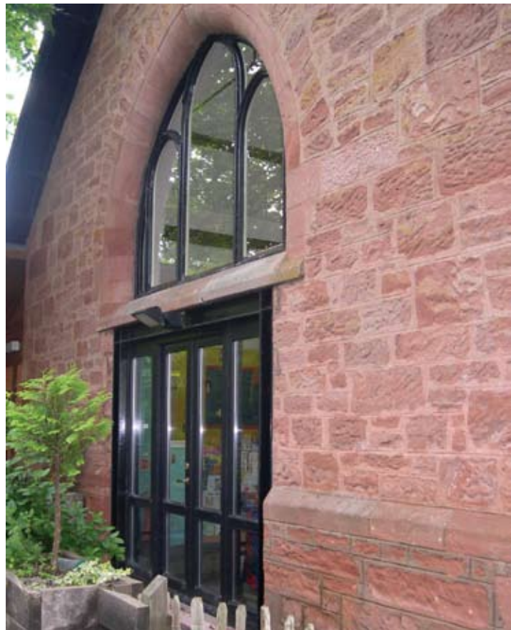
Illus 1.7 New glazed opening formed below an existing window in this gothic sandstone rubble church hall (1898) listed Category C(S) converted to community play group facility. (Photo: D Urquhart).
