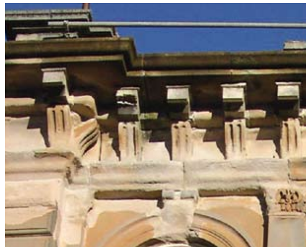
Illus 2.3. An example of inappropriate replacement elements is illustrated on this B listed building. Stone brackets supporting the stone cornice have been replaced with reinforced precast concrete brackets. The reinforcement is corroding creating a risk of falling masonry. An original stone balustrade supported on the cornice has been removed. (Photo: D Urquhart).
