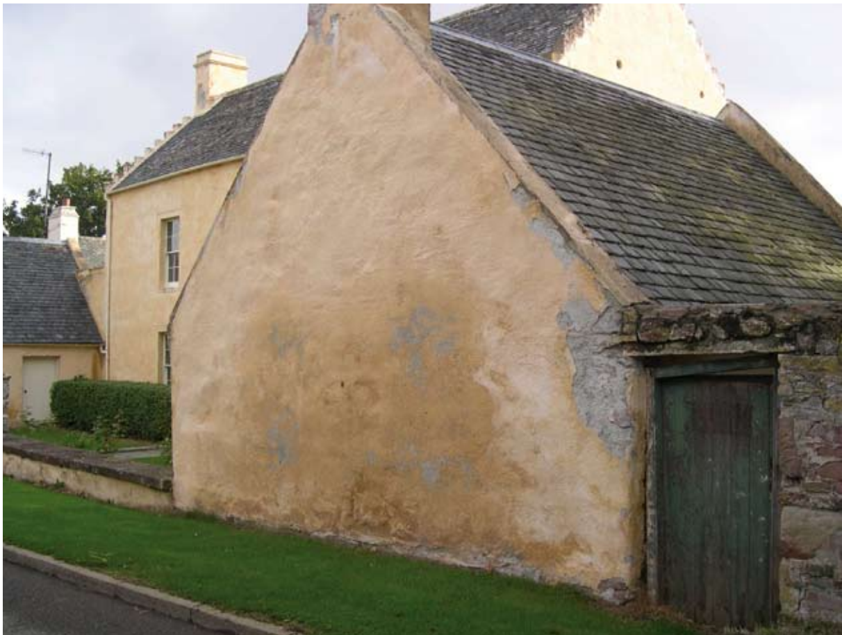
Illus 3.12(a) Recent lime coating showing exceptionally high moisture loading in the wall due to water penetration at roof level and to moisture from the ground. (Photo: D Urquhart).
