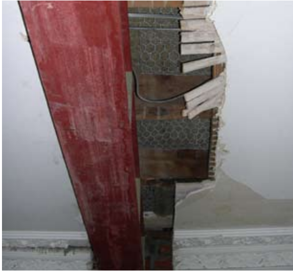
Illus 2.5 This early C19 listed Category B, former bank building, has been disrupted internally to accommodate conversion into two-bedroom apartments (Photo: D Urquhart).
