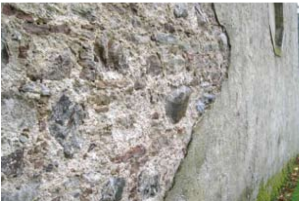
Illus 3.13 Typical failure of hard cement render on a soft mortar rubble wall. (Photo: D Urquhart).
