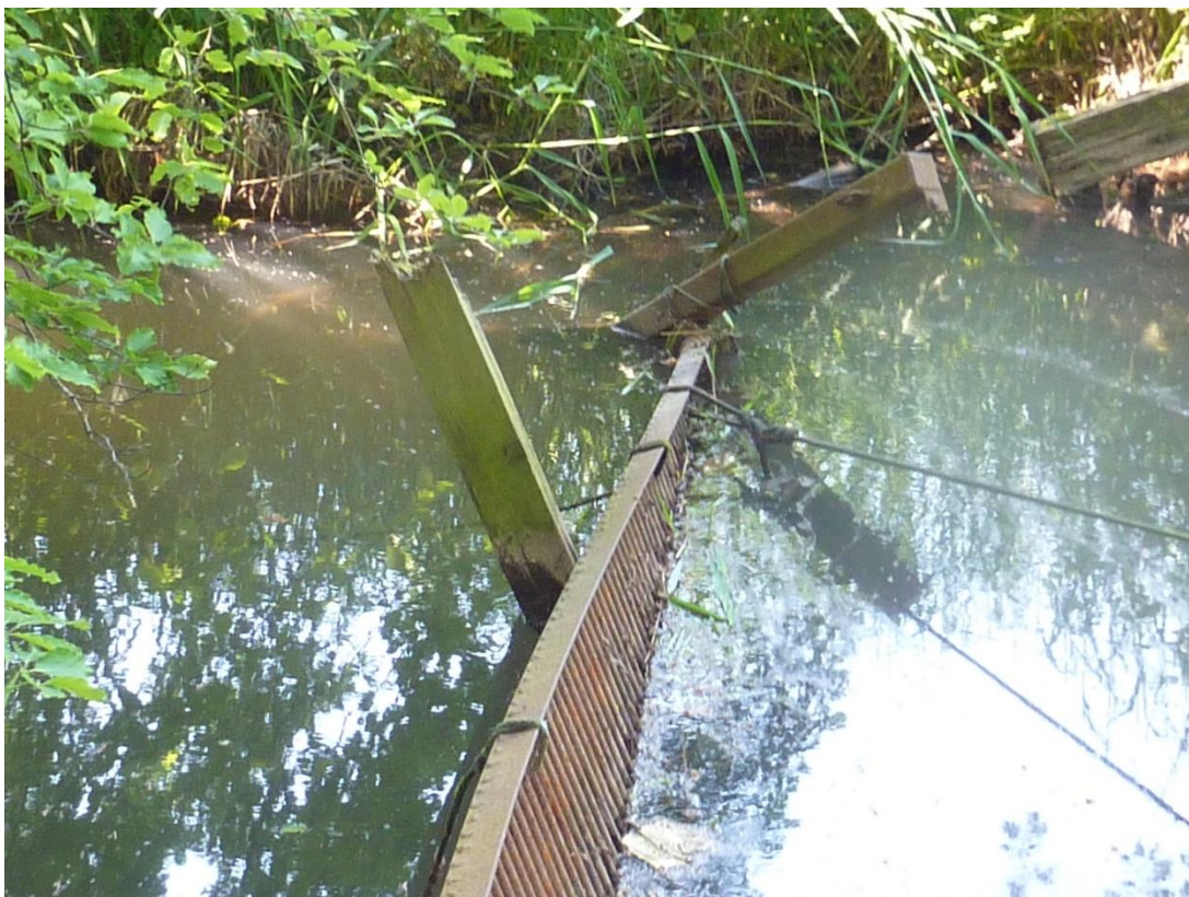
Intake water grate – awaiting repair
