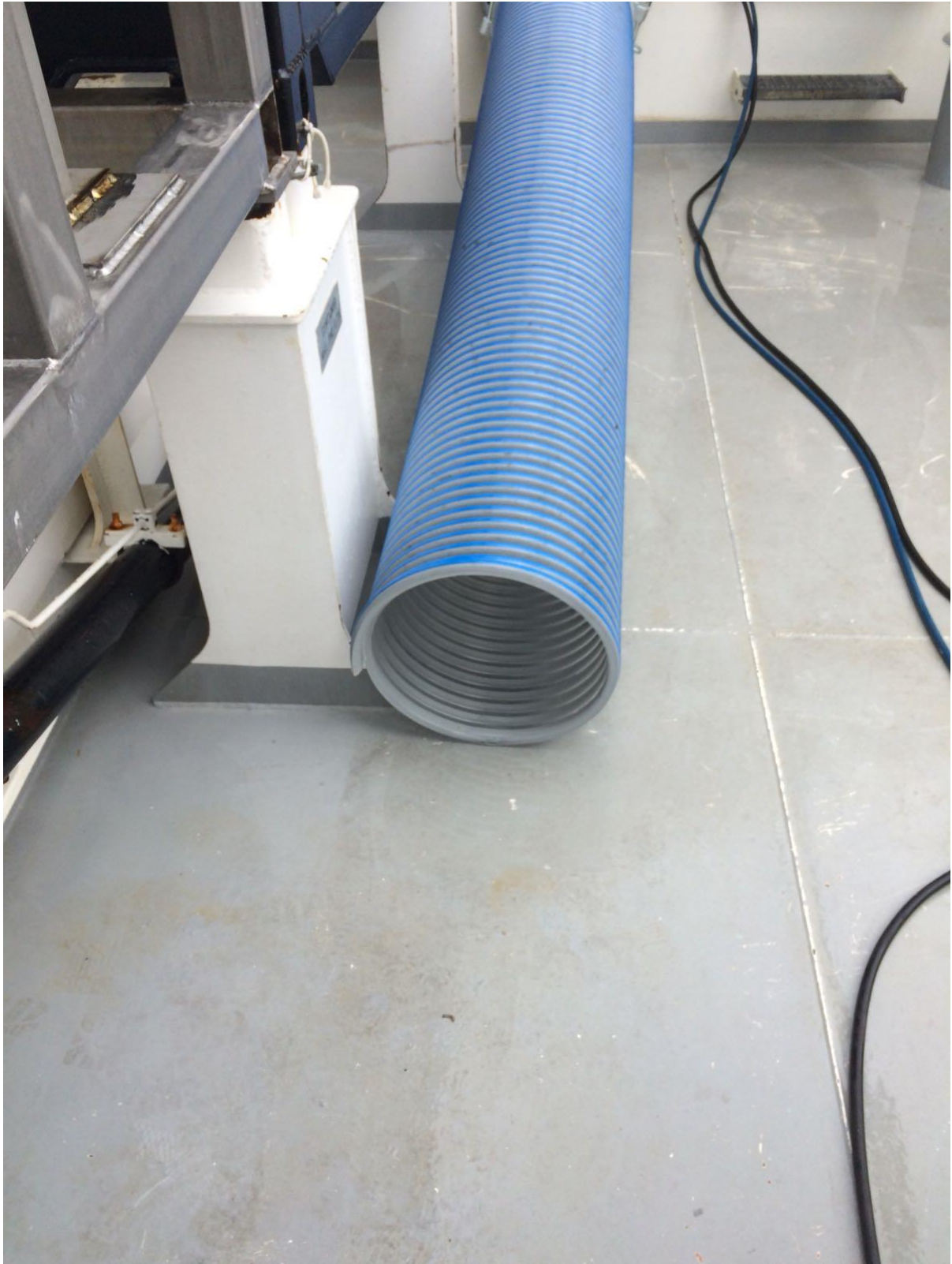
Photo 1: Split pipe in situ
